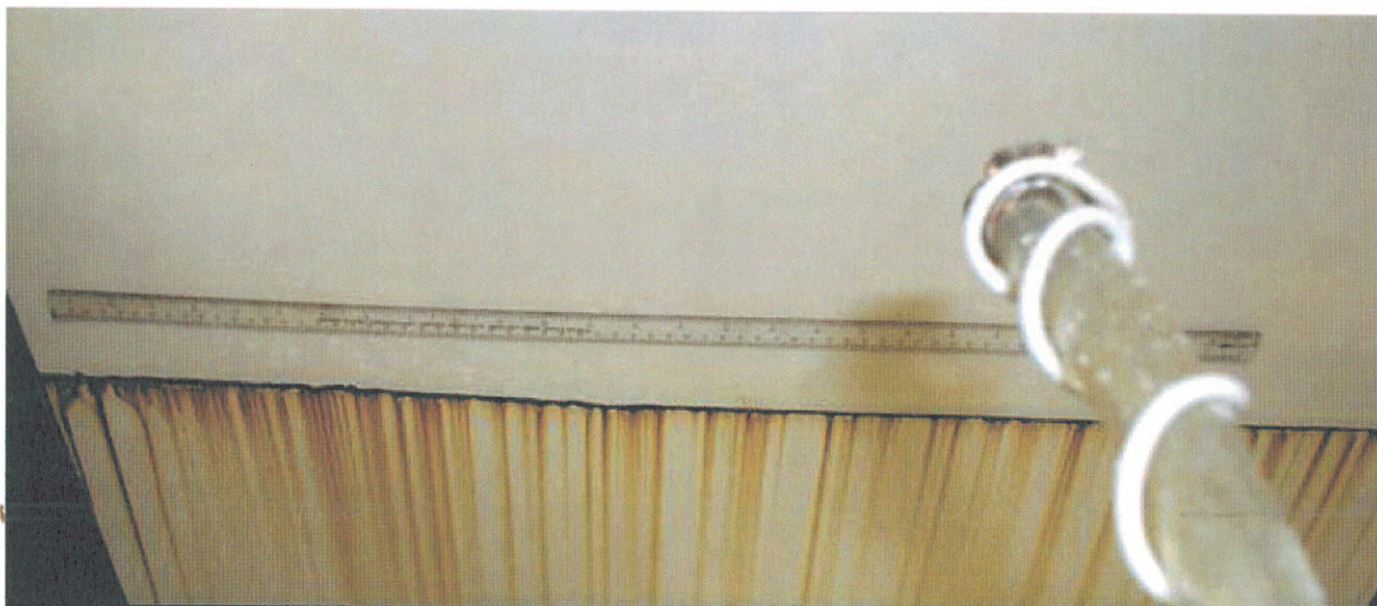
Figure 14 - Control panel appearance (Experiment Three)
